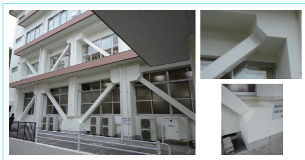
Development of low-cost seismic retrofitting technology by concrete filled steel tubular brace acting in compression for old buildings
